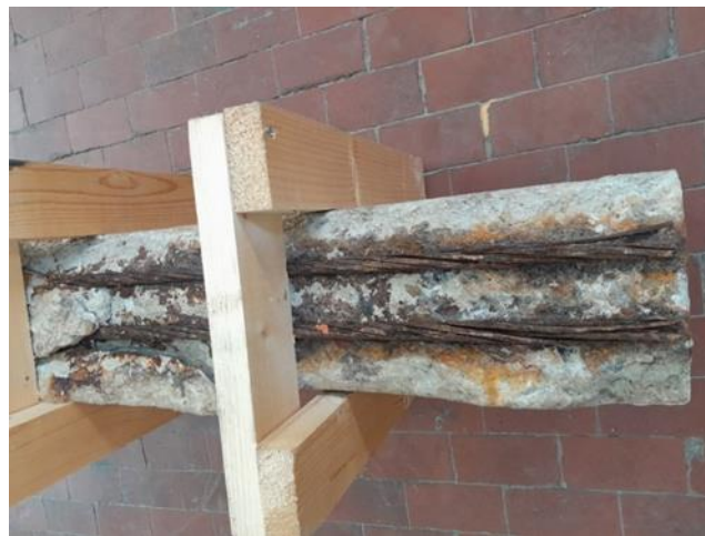
Figure 1-2 _ Chloride-induced corrosion in a prestressed concrete (PC) beam
