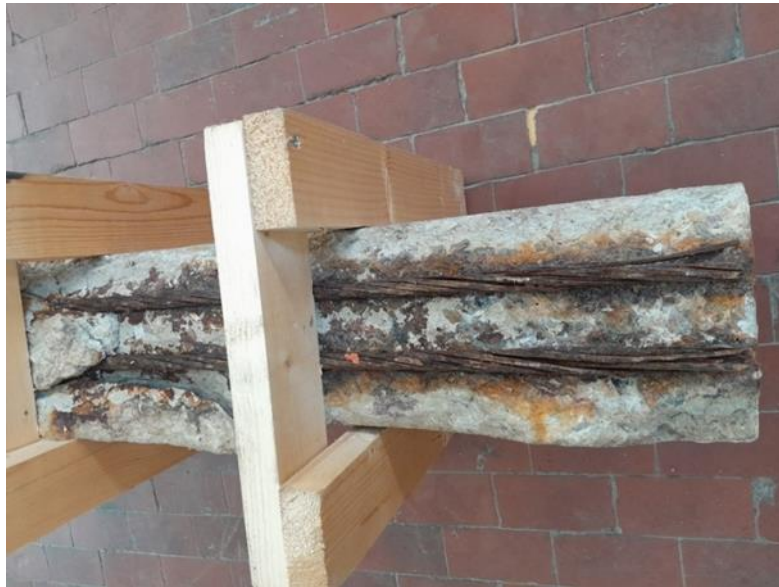
Figure 4-3 _ presence of corrosion on the strands and surrounding concrete after splitting failure, Specimen BE1-test1, this part had been at the edge of the beam resulting more exposure to corrosion
