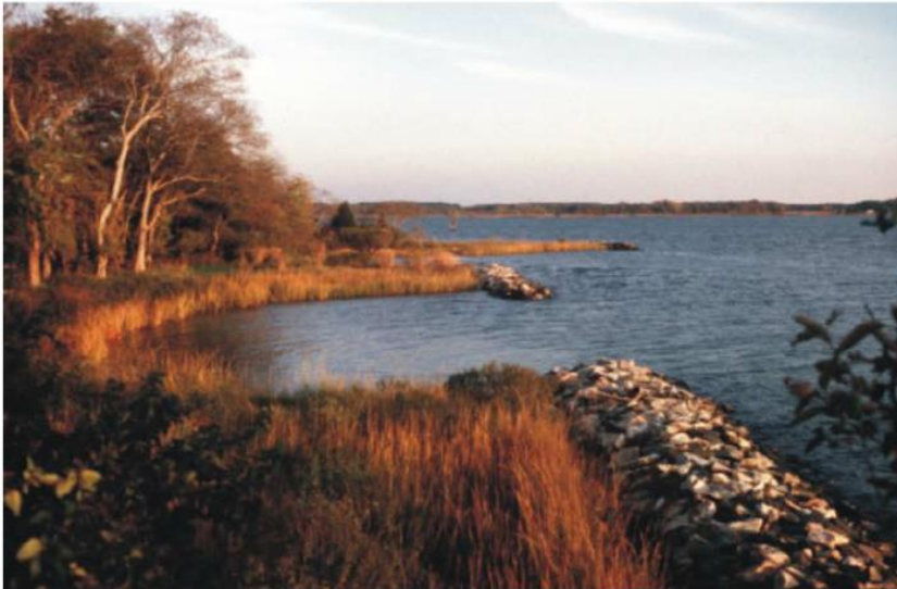
Figure 10 Stone sill connecting breakwaters with sand fill and marsh implantation on Choptank River, Talbot County, MD, just after construction and 5 years post-construction ( Byrne, 1999 )
