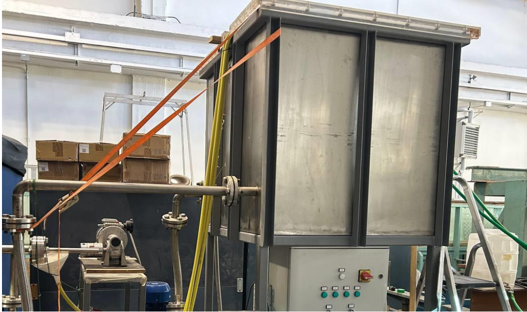
Figure 2: Tank for water storage
