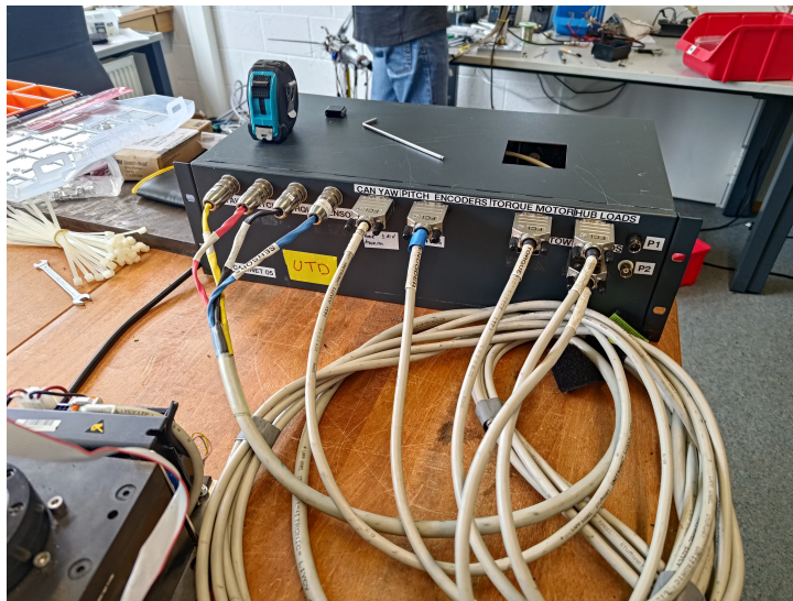
Figure 4.4: Bachmann cabinet with connections
