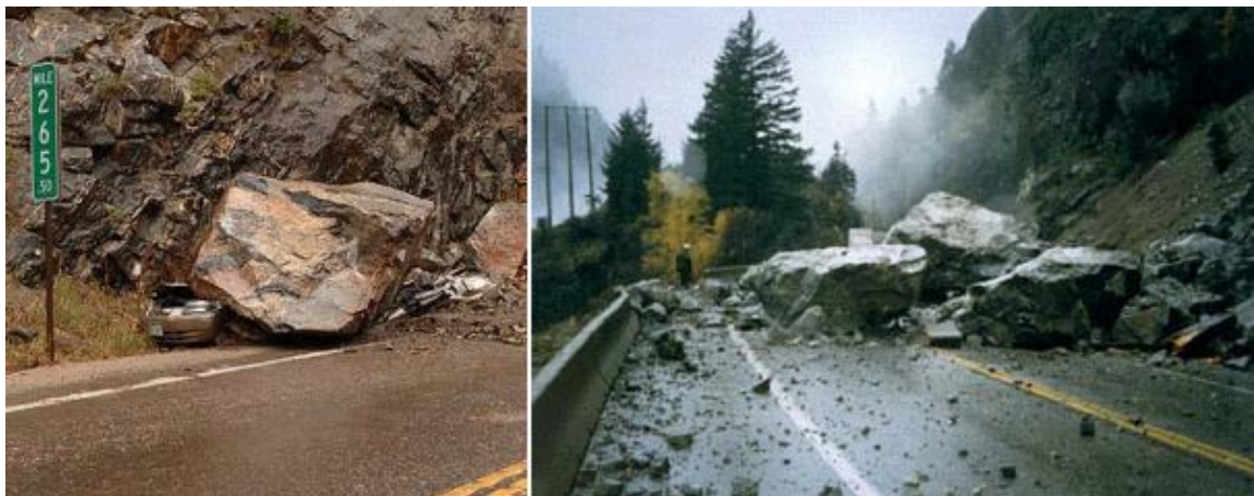
Figure 1.1.1 Damage due to RockFall
