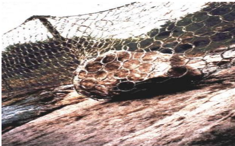
Figure 2.2.5 Geobrug ring net shown restraining a boulder. These nets can be designed with energy absorbing capacities of up to 2500 kNm which is equivalent to a 6 tonne Boulder moving at 20 m per second
