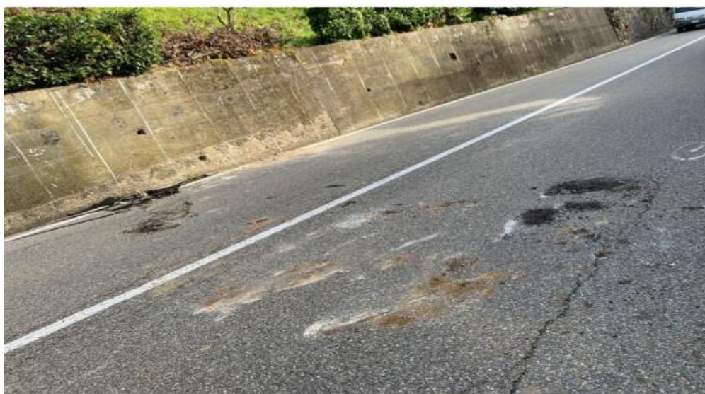
Figure 3.1.4 damage to the road surface by rockfall
