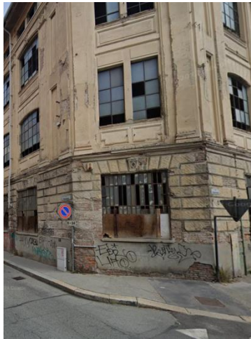
Figure 4: Broken façade of Turin
