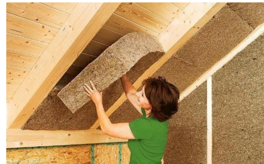
Fig 74 – Industrial hemp non-woven batts being installed as a non-toxic insulation for walls and ceilings, Source – What Is a Hemp House? | LinkedIn
