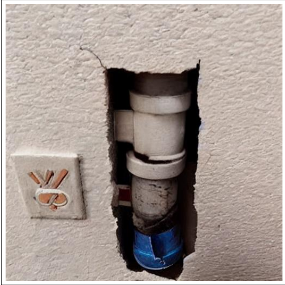
(a) Generated Image for 'Broken Pipe' category
