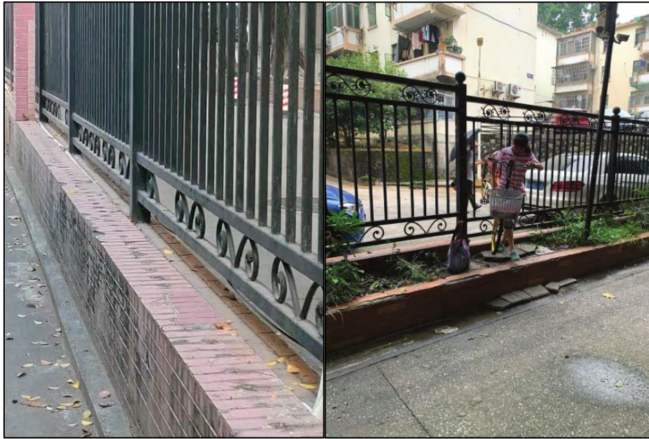
Figure 4-7 The photo on the left shows the current state of the two boundaries, and the photo on the right shows residents walking through the holes in the fence (Source: The left is photographed by the author, the right is from Reference[42])
