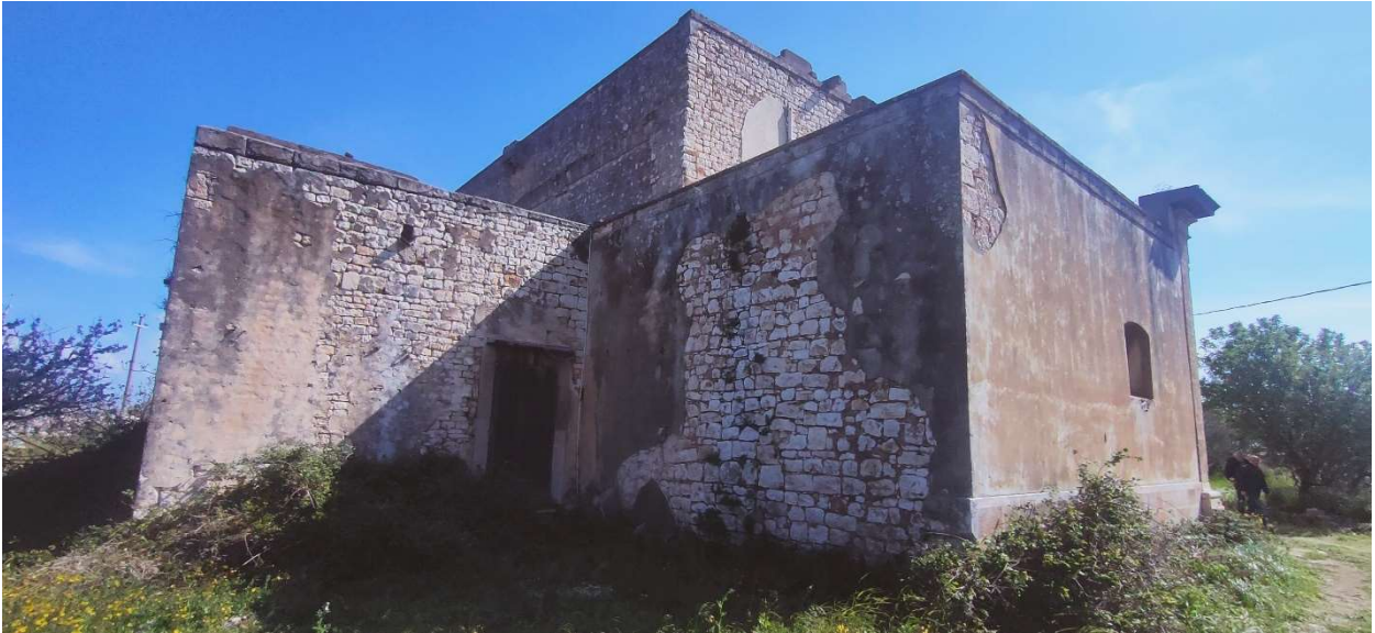
Photo 5-16: The wearing of the plaster due to weathering is evident.
