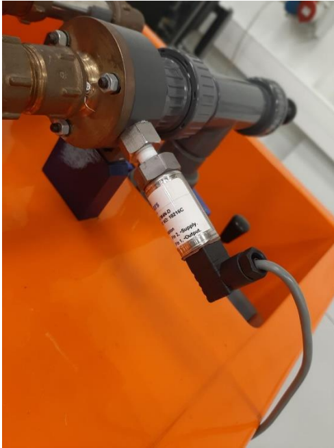
Figure 15 A pressure sensor installed at the end of the second pipe
