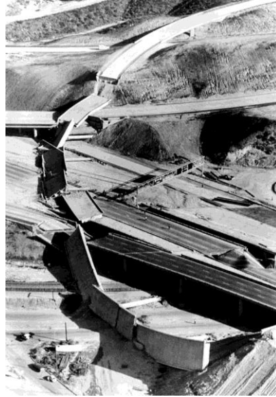
Fig 1.8. Curved bridge collapse due to 1971 San Fernando earthquake
