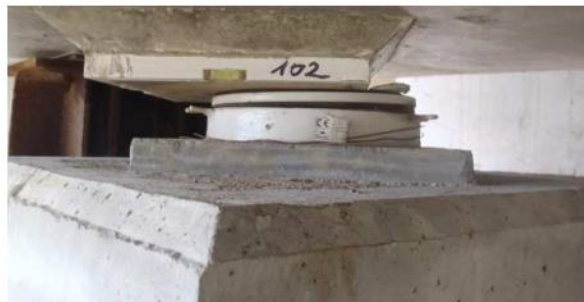
Fig.1.5. Excessive displacement of bearing plate
