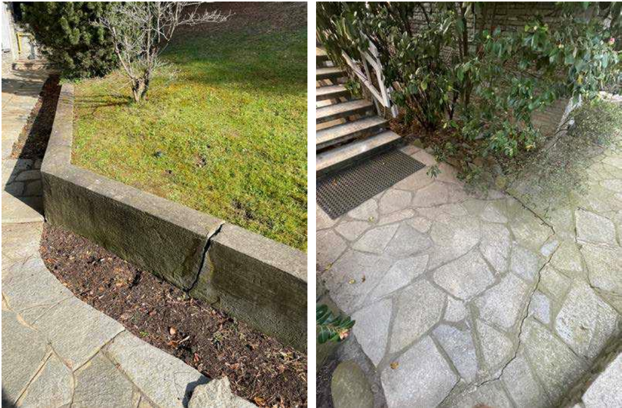
Figure 5.2 Wall and pavement cracks.
