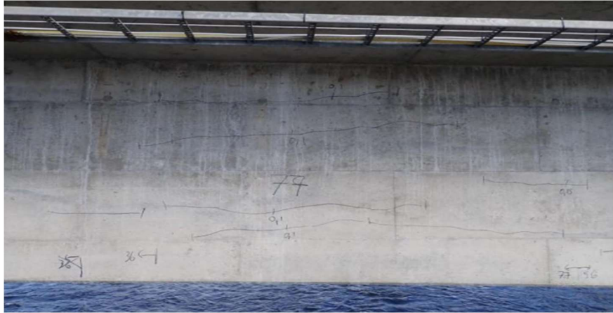
Figure 15-Crack pattern at section 77 in Figure 5 (the 1/4-point) where joints of the prestressing reinforcement are situated. There are five cracks of width 0.1 mm, but they are hard to see for the naked eye.
