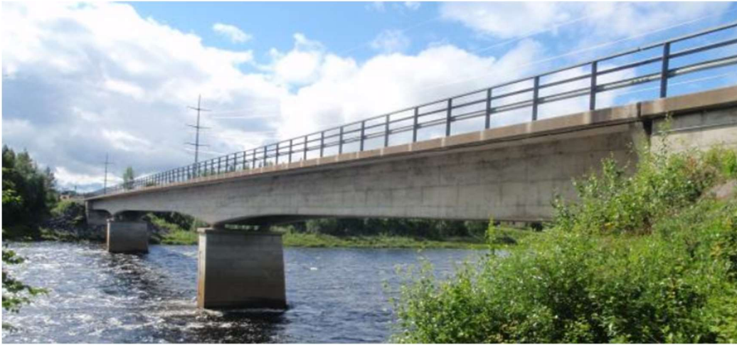
Figure 11-Prestressed Concrete Bridge over Torne River at Autio built in 1963 with three spans and a total length of 134.8 m. View towards SE.
