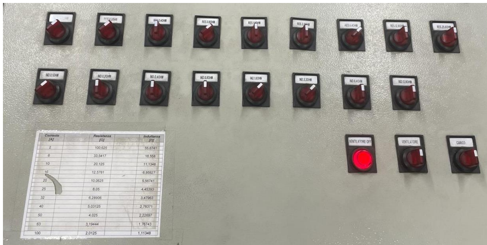
Figure 4.3: Load switches console
