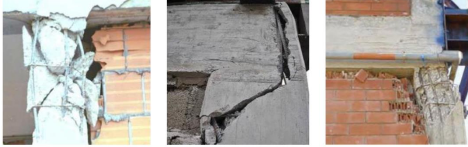
Figure 5. Local shear failure at column ends of infilled RC frames [5].
