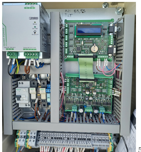
Figure 4.2: Control Unit of the Parabolic Dish
