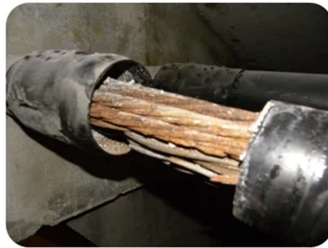
Figure 20 Corrosion in Tendons
