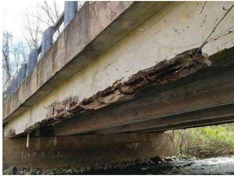
Figure 21 Concrete spalling due to corrosion
