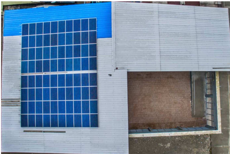
Figure 147. Photovoltaic modules in roof of Cerchocó. Source: Aristizabal, 2023.
