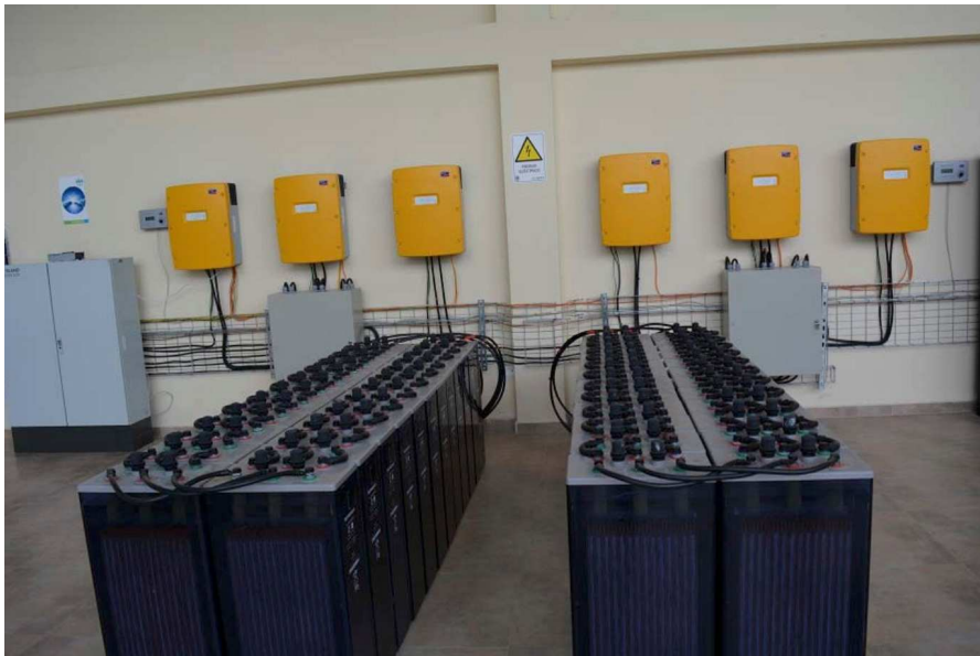
Figure 146. Battery system in Cerchocó Source: Aristizabal, 2023.
