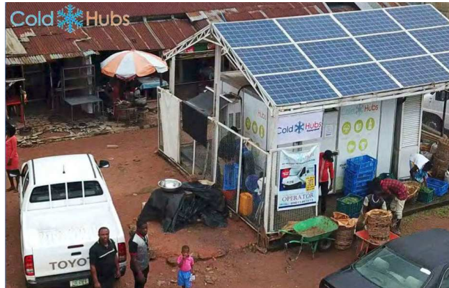
Figure 45. Micro-grid project Source: IPSE, 2022.
