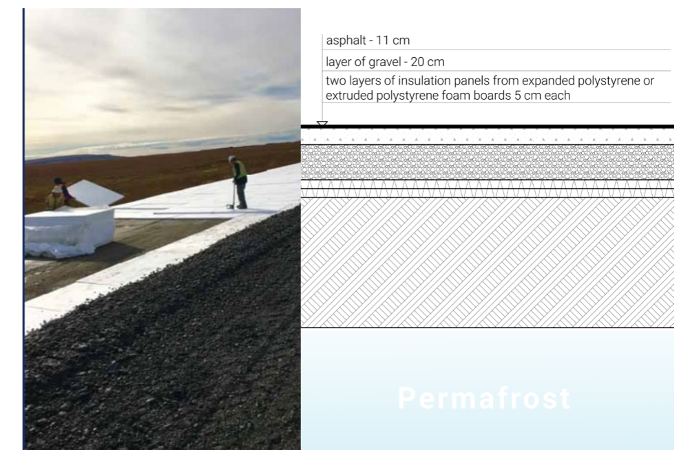
Figure 71 (on the left): a photo shows the road construction with the use of foam boards to preserve permafrost (photo is taken from https://dot.alaska.gov/traveltopics/building-in-permafrost.shtml )
