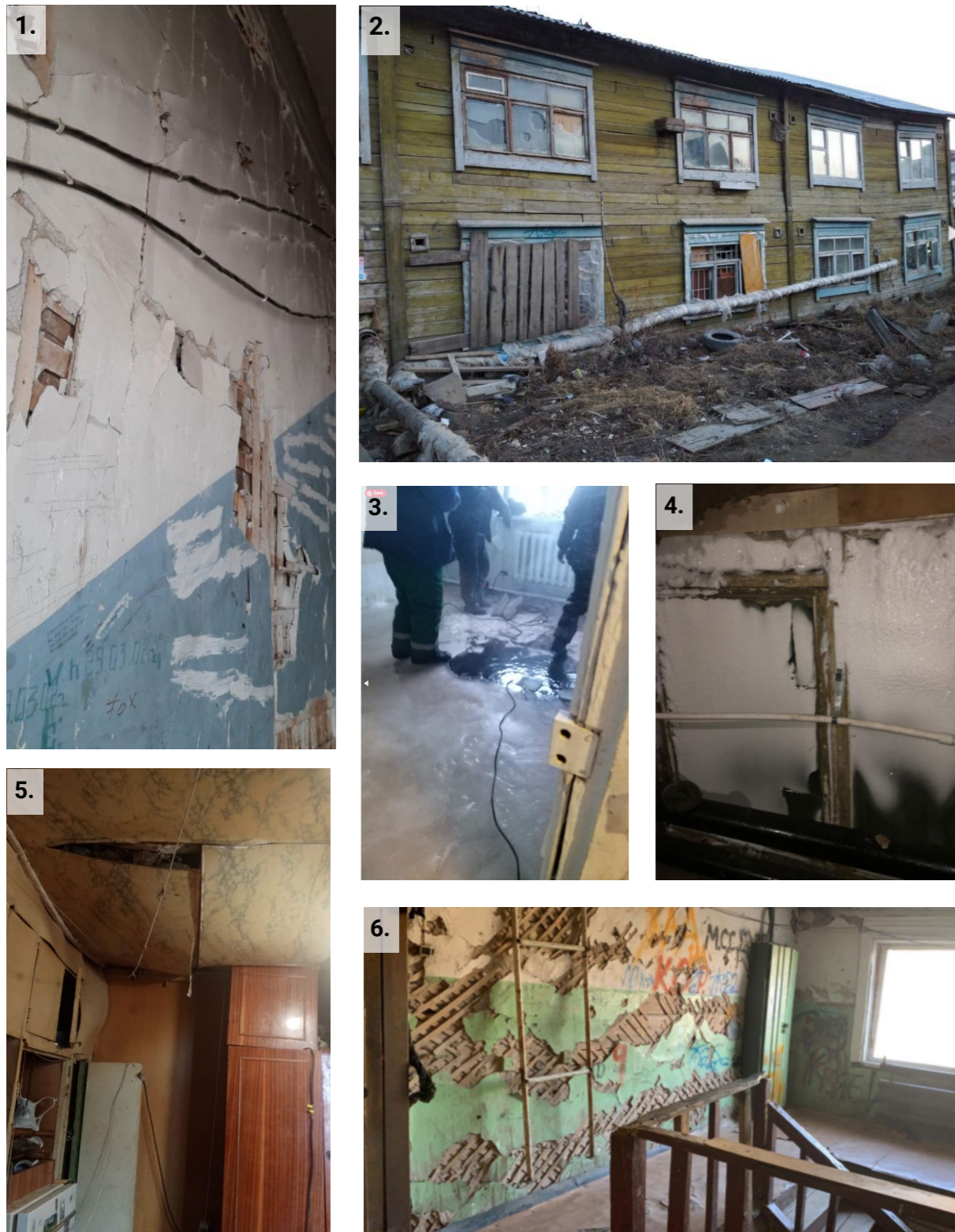
Figure 6: Examples of the buildings that have received the emergency state and after locals will receive new houses and leave the building the structure will be demolished. 1 - the condition of the load-bearing wall; 2 - the house is gradually sinking into the ground due to heat losses, permafrost thawing, and following land subsidence; 3 - due to the land subsidence the house sink into the ground, the ground floor is flooded and with winter time turned into the ice; 4 - the inefficient building envelope creates the condensate on the walls, that turns into the ice and snow; 5 - we can see that the structure of the house is not capable to bear loads, and the ceiling is basically held by the wardrobes.; 6 - the interiors of the house, fallen plaster allows us to see the structure of the wall (Photos source: https://news.ykt.ru/article/120223 ).
