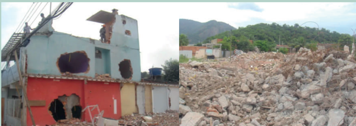
Fig. 106 Demolition of the houses of former residents evicted from Vila Autodromo, Rio
