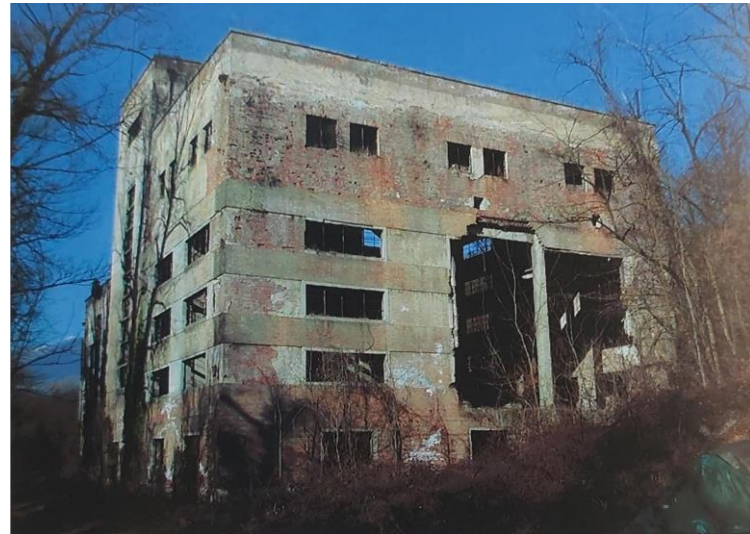
Figure 51: Thermoelectric power plant, the state of abandonment. 209
