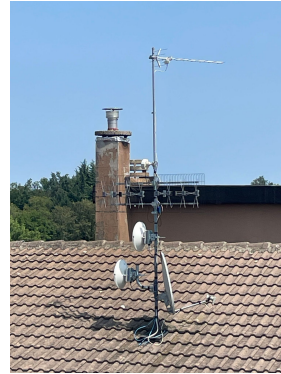
Figure 3.1: a) An hybrid node in Villadeati (AL), b) A CPE on the rooftop
