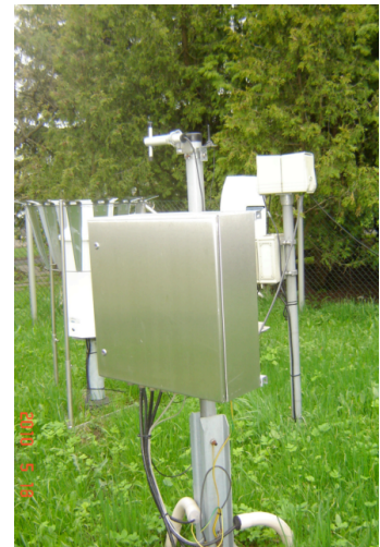
(f) Data collection, processing and transmitter unit
