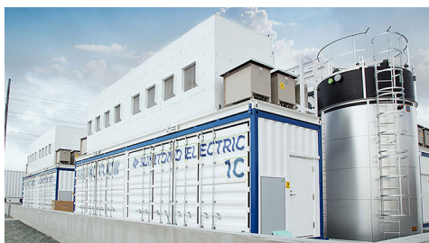
Figure 10: Vanadium Redox Flow Batteries
