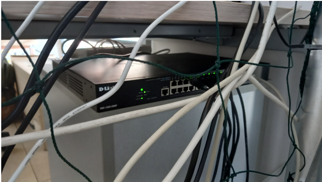
Figure 2.17. Representation of the switch used to link every VICON camera together with the main GCS
