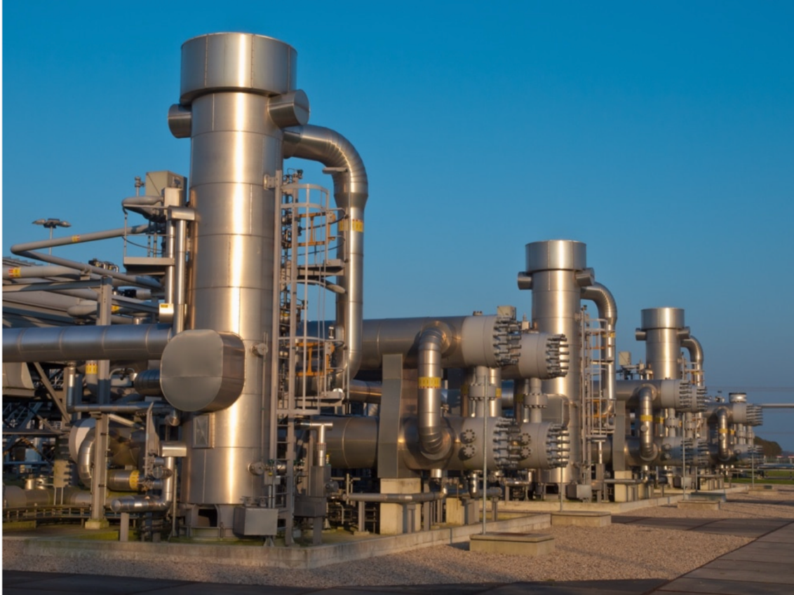
Figure 4.4 Groningen gas processing plant [44].
