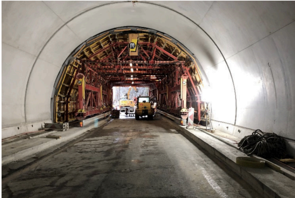
Figure 2.3-2 - FEDRO Tunnel: casting of the new final lining with a moving formwork
