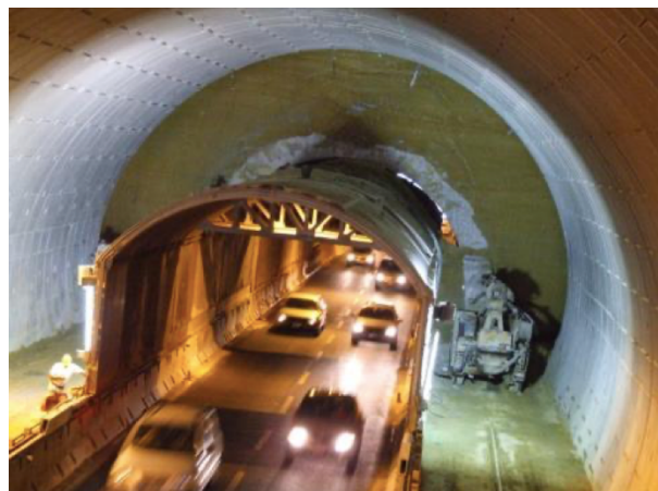
Figure 2.5-2 – Nazzano Tunnel: traffic protected by the steel protection shield while the old tunnel is being widened.
