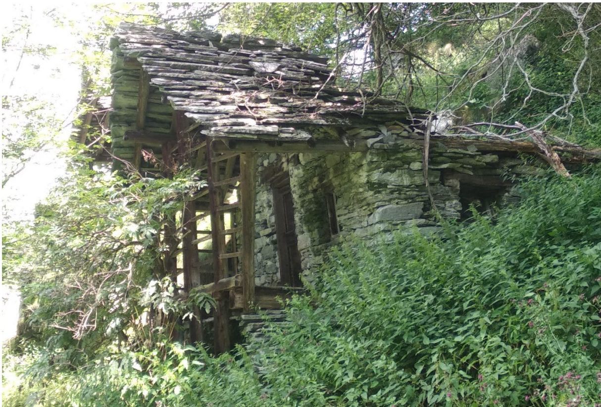
Figure 104 stadel with collapsed roof; close to Alagna (photo: Z.Miłek)
