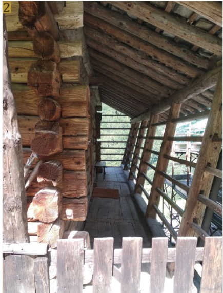
blockbau walls; 1 visible fissures in part of the house used as a storage / 2 corner connection u-shaped
