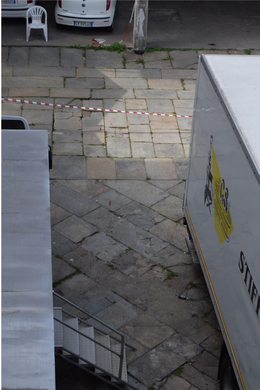
Figure 56 - Detail of the flooring of the southern area of the internal courtyard.
