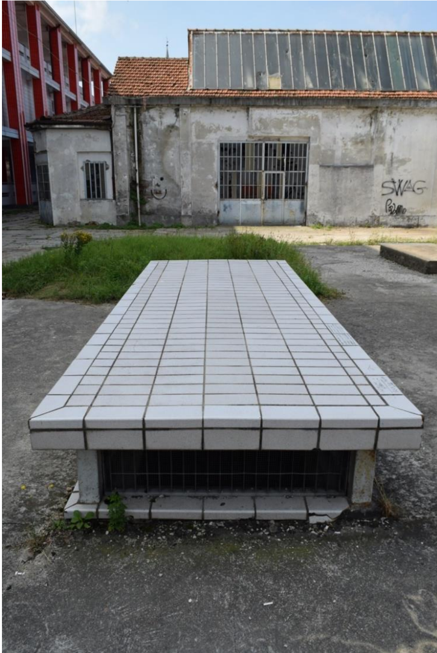
Figure 47 - Detail of the air inlets for the natural ventilation of the underground parking.
