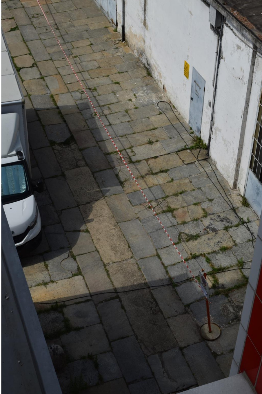
Figure 54 - Detail of the flooring of the southern area of the internal courtyard.
