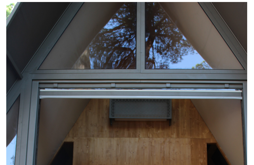
Figure 05.5.16-20: Images of the installation of the automatic door screen and AC unit Source: Pictures taken by the author of the thesis
