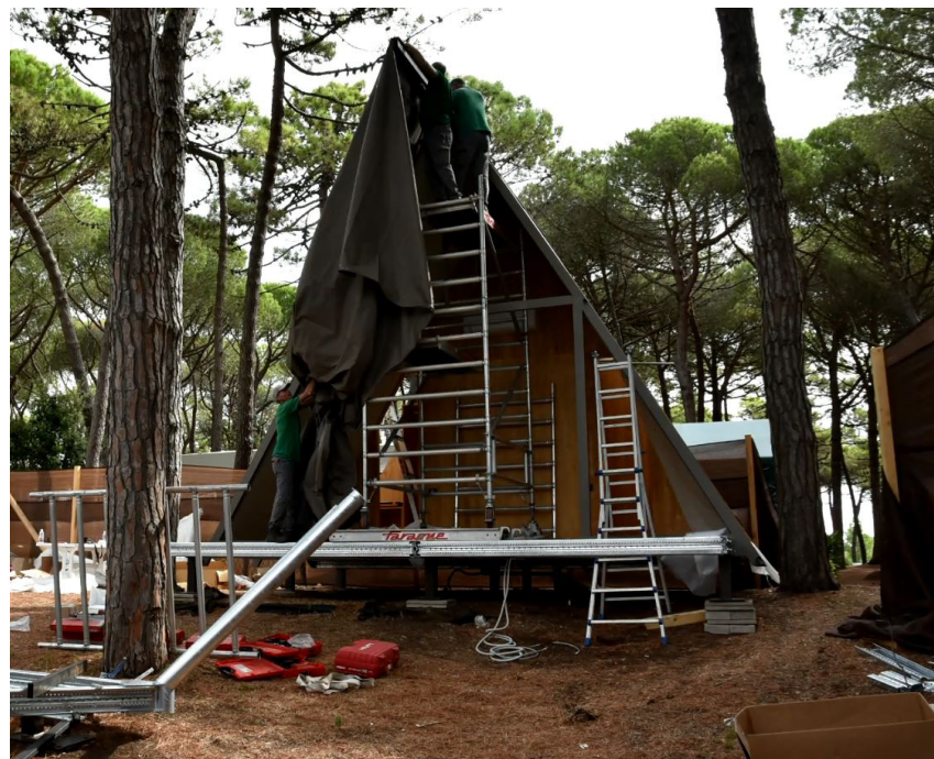
Figure 05.5.11-15: Images of the assembly of the prefabricated steel frame and installation of the envelope inner and outer fabric layers Source: Pictures taken by the author of the thesis
