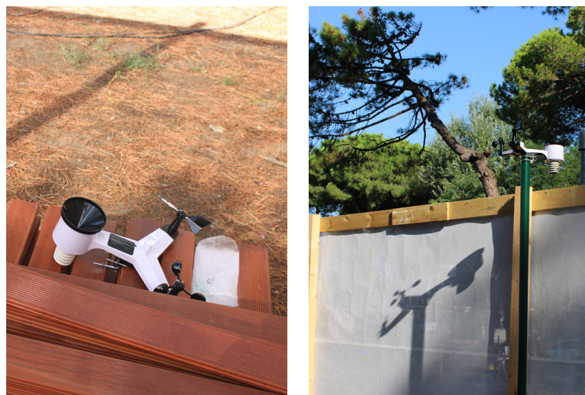
Figure 05.5.21-24: Images of the installation of the platform deck - installation of the micro-climatic survey station Source: Pictures taken by the author of the thesis
