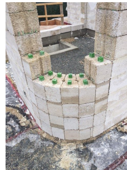
Figure Pf27-28: Just BioFibre - Harmless Home project - building blocks - construction process Source: https://justbiofiber.com/projects/
