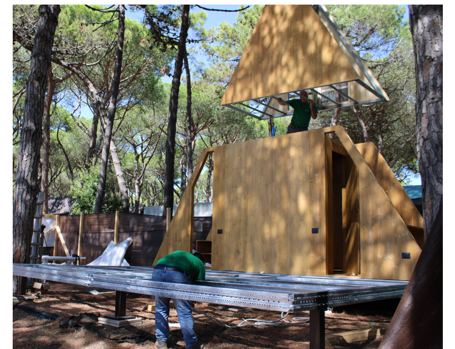
Figure 05.5.6-10: Images of the installation of the prefabricated bathroom and dressing room module Source: Pictures taken by the author of the thesis
