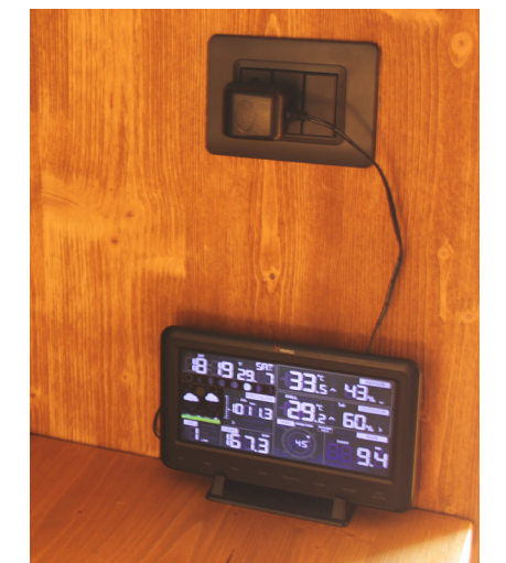
Figure 05.6.17: ICOMAC27 - Micro-climatic station control panel installed on site during the site survey. Source: Picture taken by the author of the thesis
