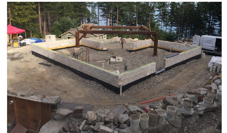
Figure Pf29: Just BioFibre - Serenity Home project - building blocks - construction process Source: https://justbiofiber.com/projects/
