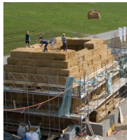
Figure St04: Atelier Werner Schmidt - Gartist GmbH - straw bale roof structure Source: https://www.atelierschmidt.ch/gartist-bubikon
