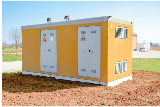
(a) Secondary substation in Italy.
