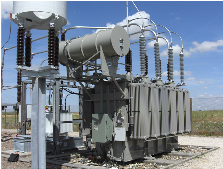
Figure 1.2: HV-to-MV transformer in Italy.
