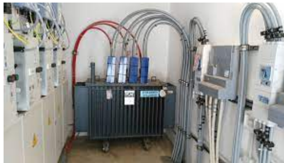
(b) MV-to-LV Transformer.
