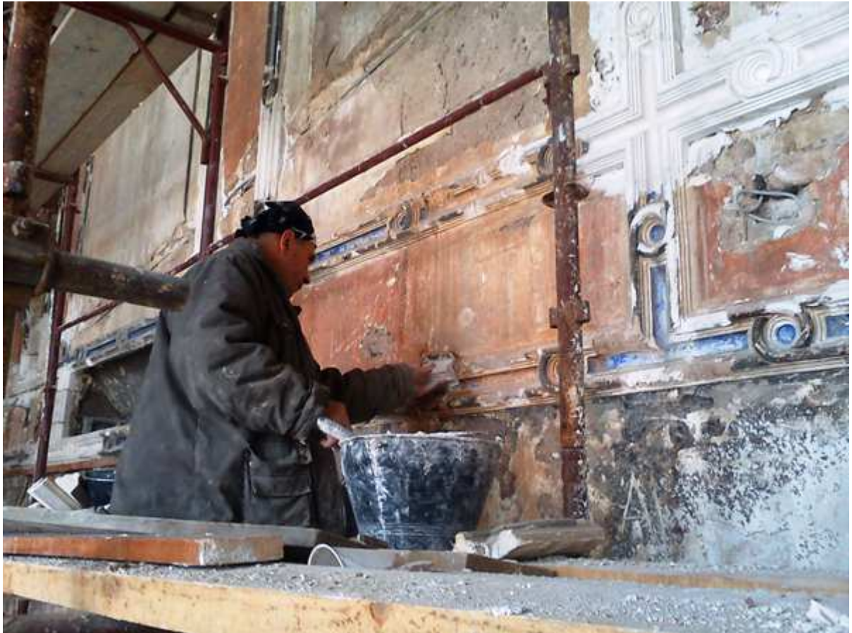
Reconstruction of missing parts of the plaster decoration in the library of "Vijecnica" in Sarajevo
