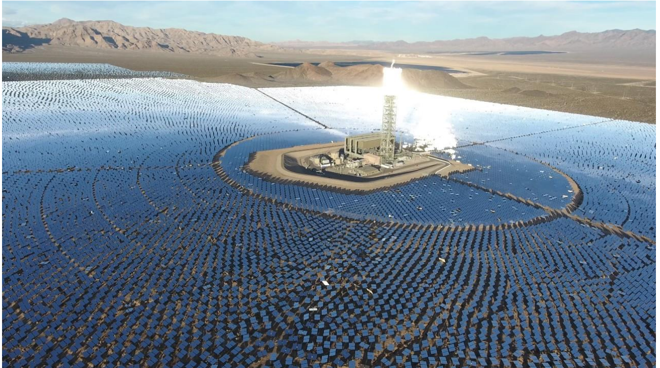
Figura 2.17 - Ivanpah Solar Electric Generating System, California [87]
