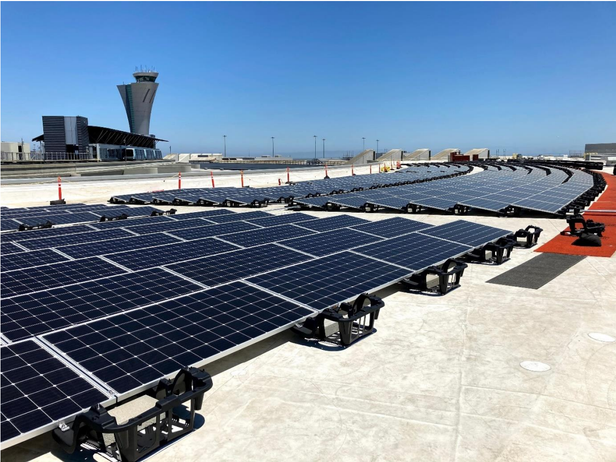
Figure 11: Sollega Inc.'s ballasted roof mounts installed into a PV system [81].
