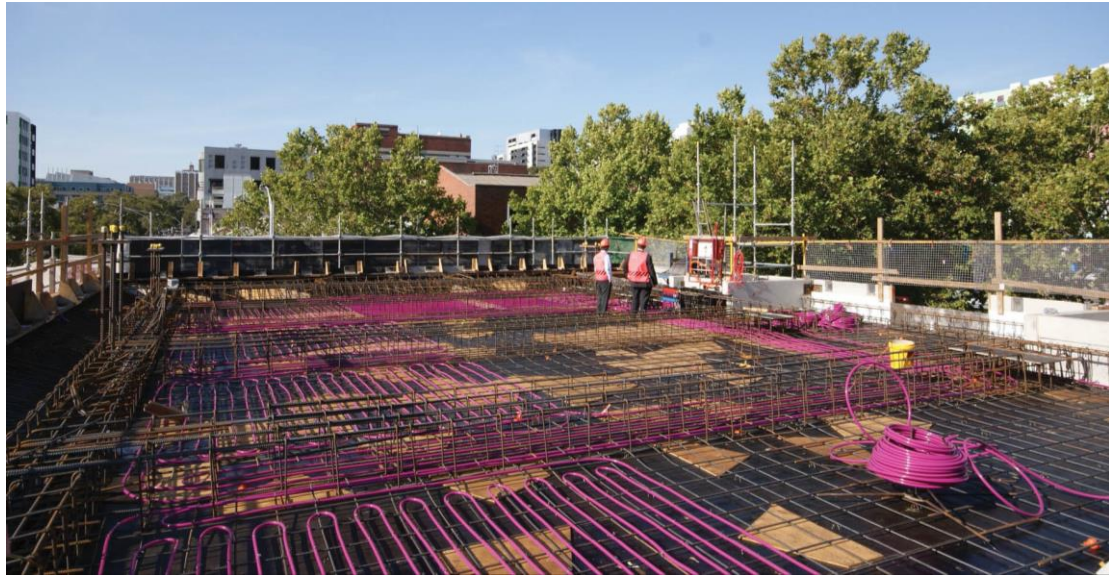
Fig 2.8 Roof heating system (Pixel building)
