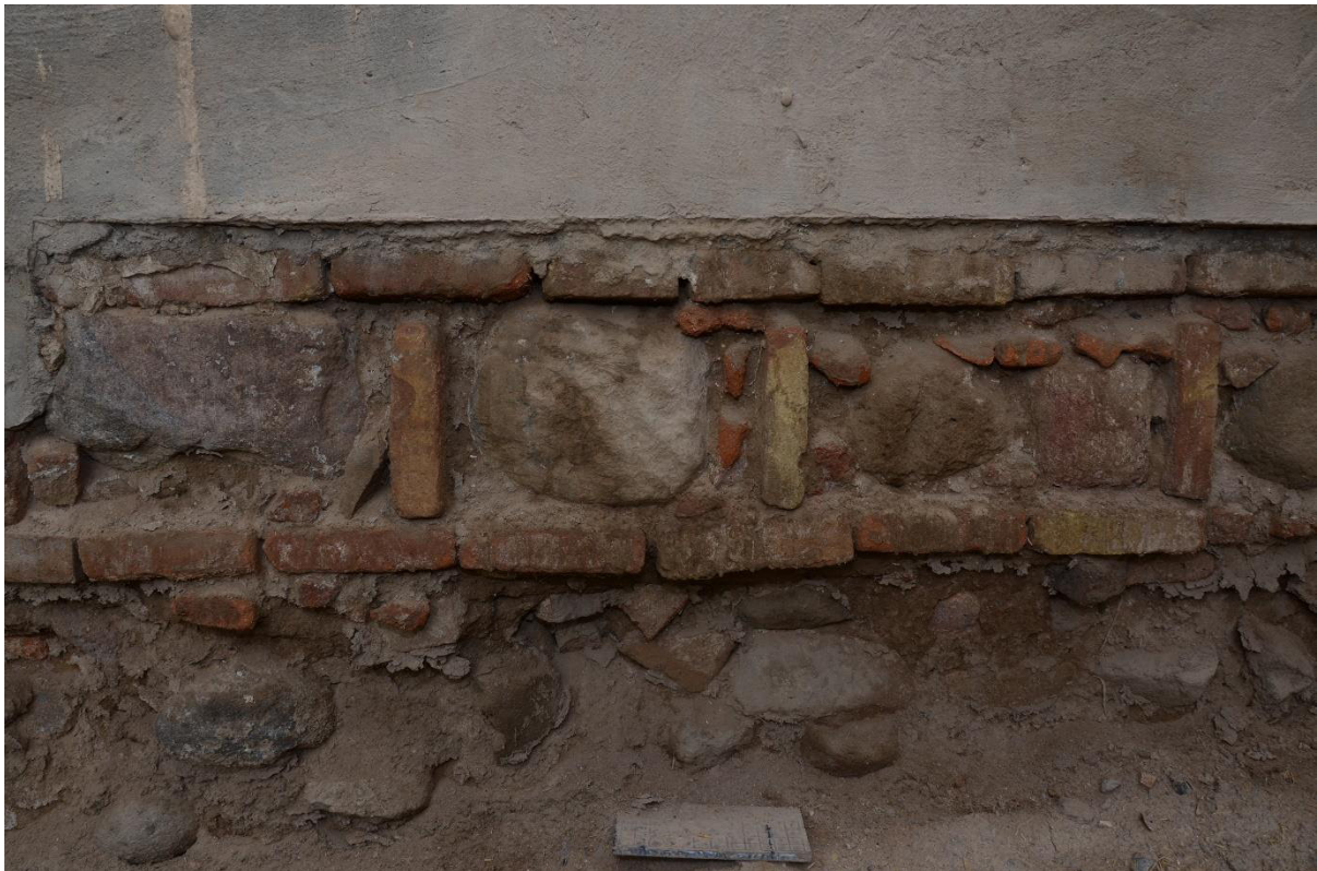
Figure 3-47: The foundations of the dwellings were composed of stone and brick. (Photo by Arsalan Chabok)
