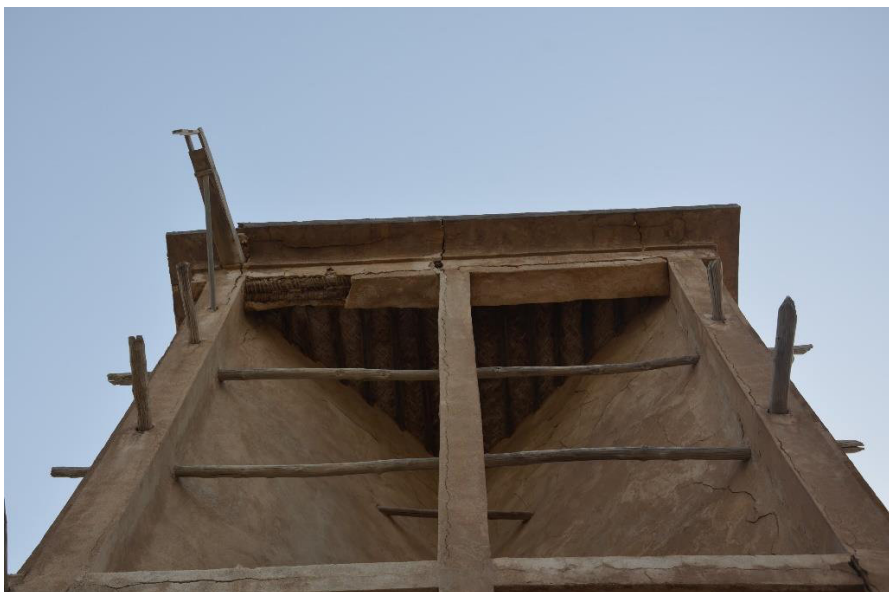
Figure 3-34: Increasing magnification of each successive detail of the wind tower (Photo by Arsalan Chabok)
