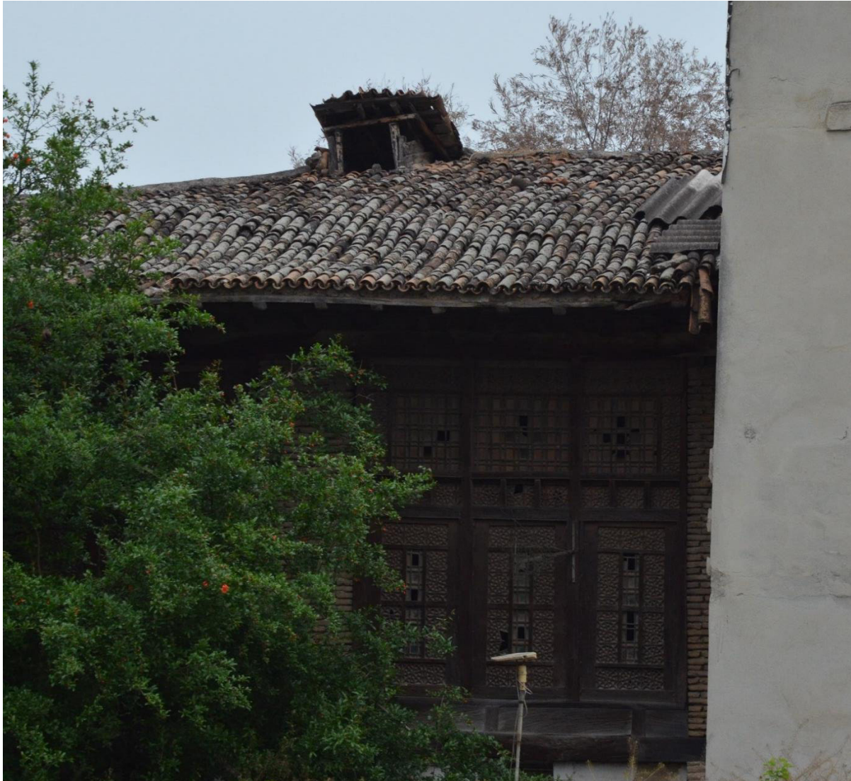
Figure 3-16: Sloping roof with cover of pottery also opening for ventilation. (Photo by Arsalan Chabok)
