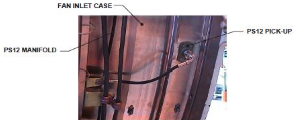
Figure 1.6: CFM56 - Pressure pick-ups, [5]
