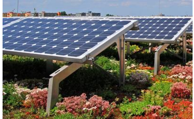
Fig. 60 Solar panels integrated with green roof Retrieved from ZinCo, (2022)
