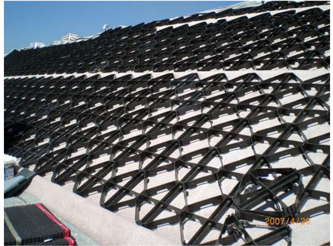
Fig. 55 installation of ZinCo-Georaster®-elements for reinforcing the sloped green roof Retrieved from (ZinCo, 2022)
