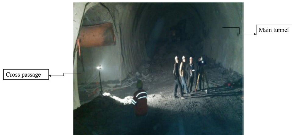
Figure 8 Example of the intersection area of a cross passage and main tunnel
