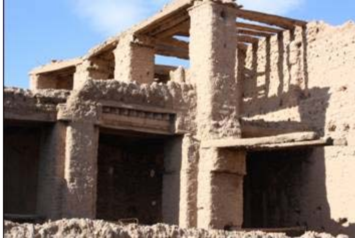
Photo of the state of decay of a traditional house
