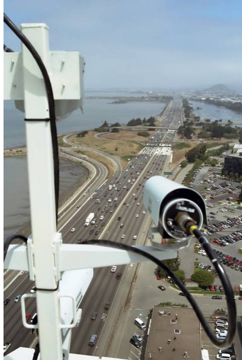
Figure 11: Camera mounted on top of a building adjacent to the highway
