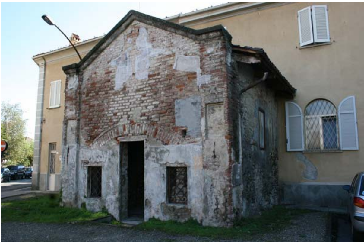
Outside of San Vito's chapel that emphasizes the degradation before the restoration interventions
