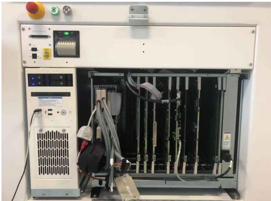
Figure 5.4 control system inside the “T100”
