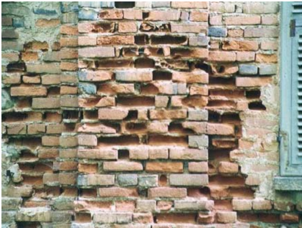
Erosion of the brick
